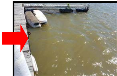
Finger Dock Missing
